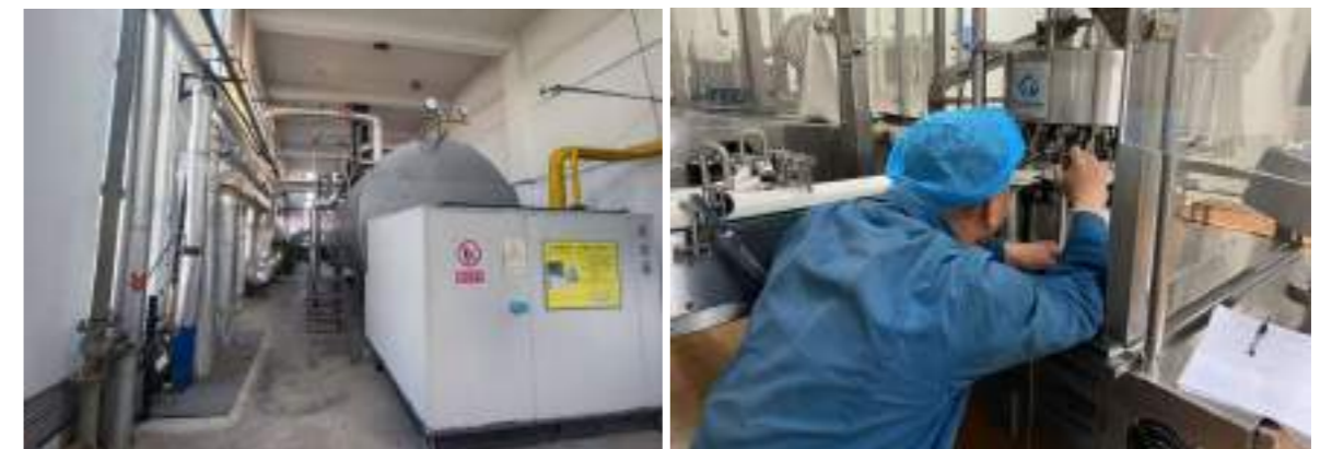
Upgraded boiler room to reduce NOx emissions
