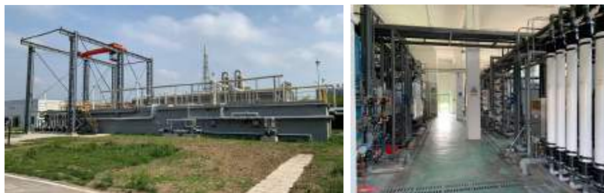
Newly built wastewater collection and treatment system
